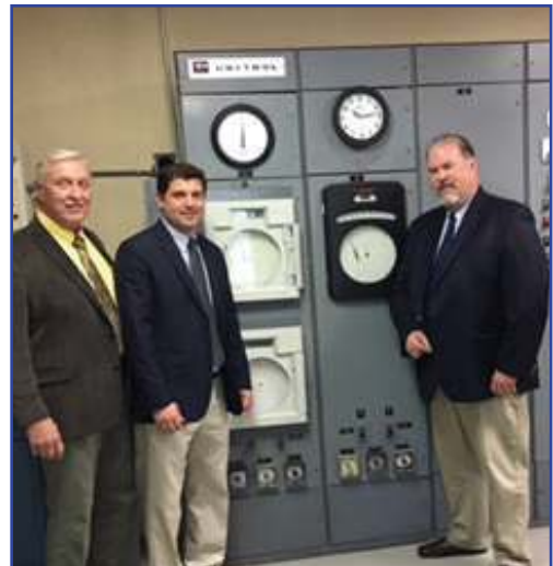
Board of Commissioners (l-r Niznik, Rich, McEvoy) at Plant No. 6 Control Panel which is to be replaced with Computerized Control System in 2017
